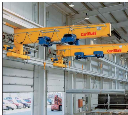
Wall Traveling Crane
